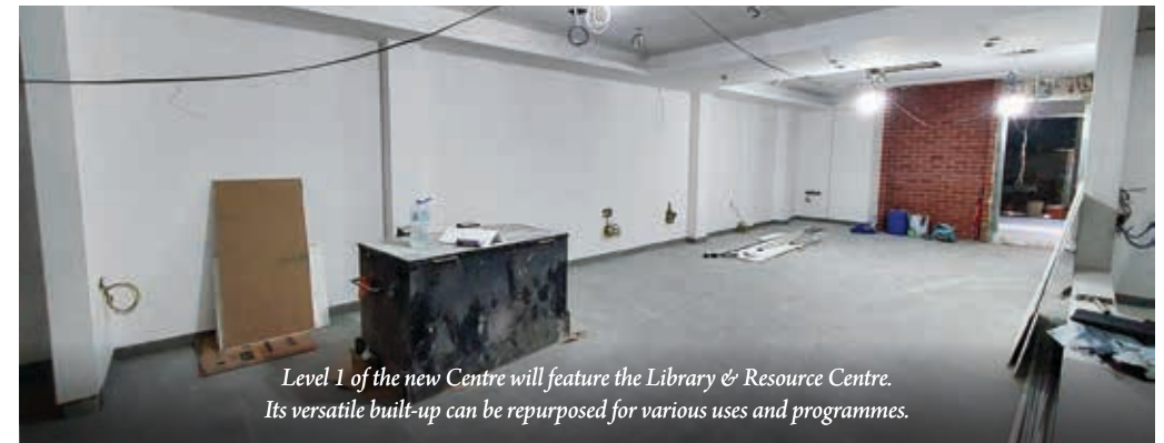
Interior work will commence soon on the new Shrine Hall located on Level 2. The expanded facility will accommodate up to 200 people, four-times its previous capacity.
